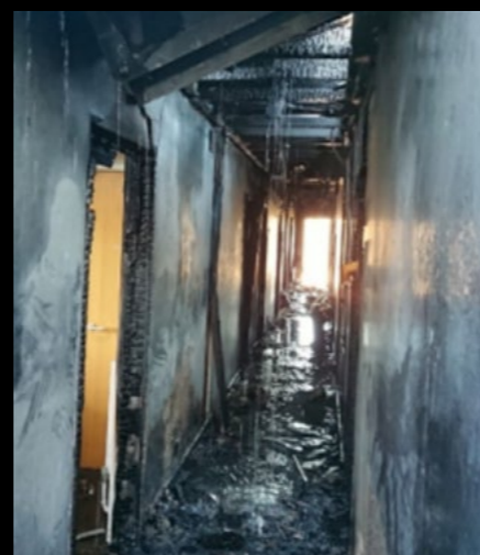
The extensive damage caused by the Boulmer SLA fire.
