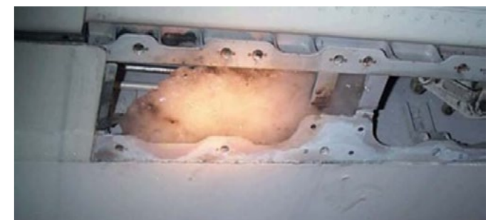
Anti-icing residue in the leading edge of the elevator trim tab
