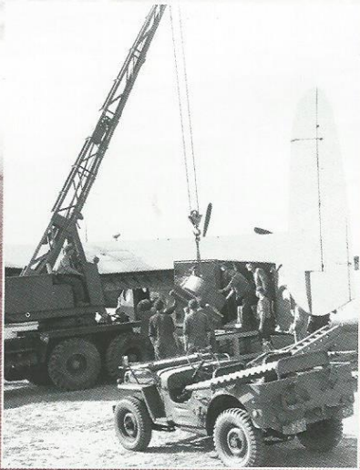
Airfield Construction 3: In Berlin even the construction plant to make improvements to the airfields had to be flown in. A steamroller is unloaded by crane through the rear door of an Avro York at Gatow.
