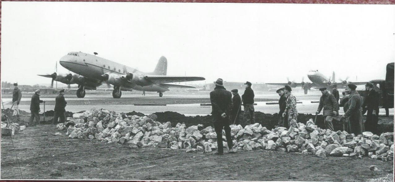
Airfield Construction 2: Handley Page Hastings taxi past German labourers working on improvements to the airfield at Schleswigland.
