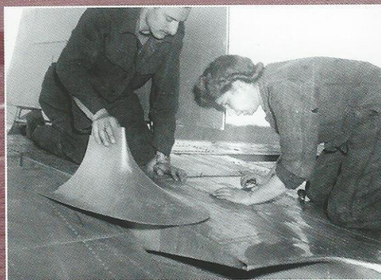
United Effort 2: RAF and WRAF fitters make repairs to the tail of a York at Wunstorf.
